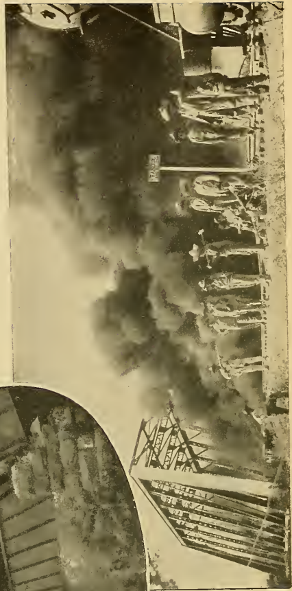
Bridges dynamited and set afire with cars of burning coal and coke. These bridges took three years to build and cost $800,000.
